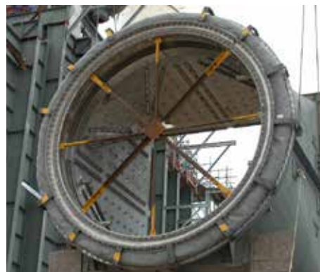
Installation of Combine-X on diffuser.
