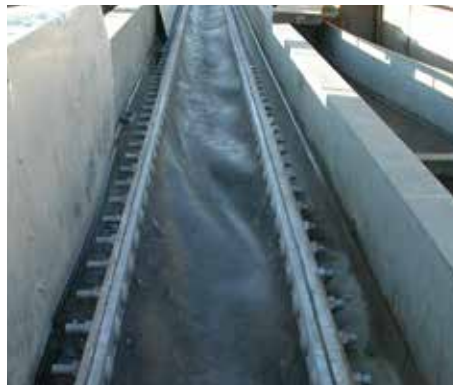
Fluachem Elastomer installed in a horizontal duct.
