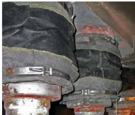
Flexgen expansion joints installed as pipe penetration seals.
